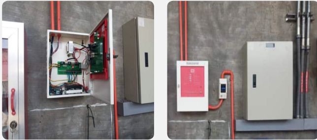
Fire Detection Alarm System (FDAS)
