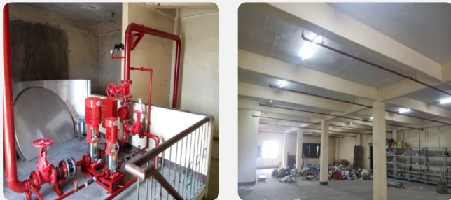
Automatic Fire Suppression System (AFSS)
